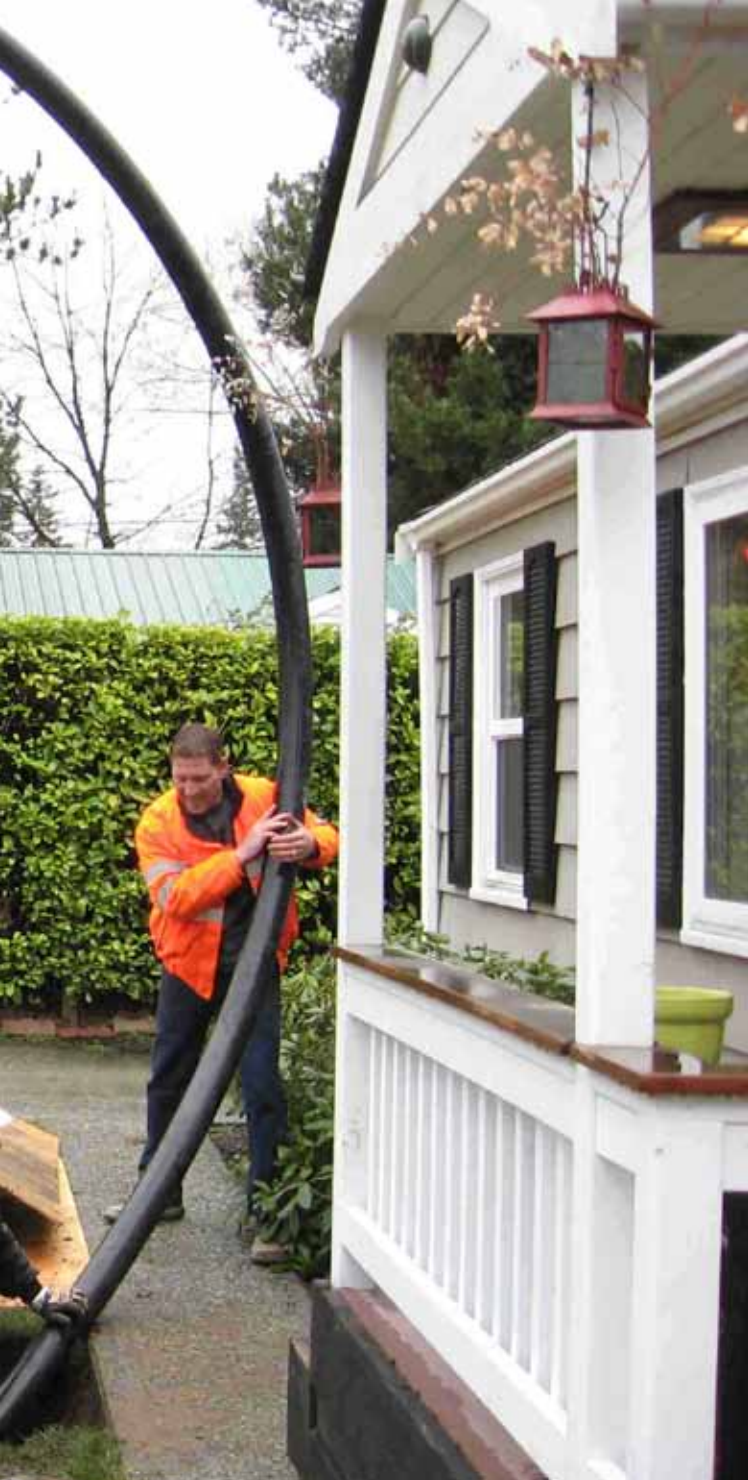
By replacing side sewers – the portion of the lateral on private property – the Ronald Wastewater District (Shoreline, Wash.) has achieved great reductions in inflow and infiltration.
